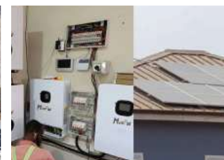
8KW solar+20KW/20KWH Off-Grid Solar System in Accra, Ghana
