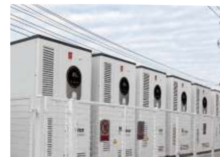
0.92MW/1.832MWH in Huzhou Tianlin Textile factory
