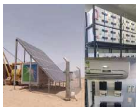
26000btu off-grid solar air conditioner system in Saudi Arabia
