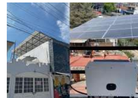
20KW on-grid solar system in Mexico
