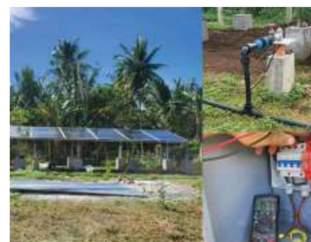
30KW solar water pump system in Myanmar
