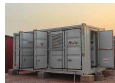
500KW+1MWH BESS project in Tanzania
