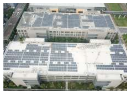
Midea Global Innovation Center Installed Capacity: 5500kWp
