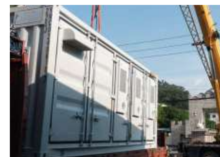
500KW/1MWH ESS in Central Africa
