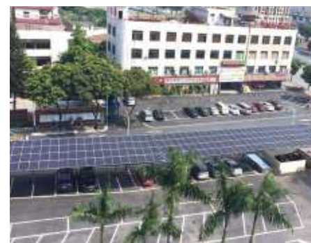
153.29KW photovoltaic carport project at Foshan Geely Plaza
