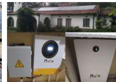
6.6KWP solar+8.5KW/10.24KWH offgrid solar system in Kenya
