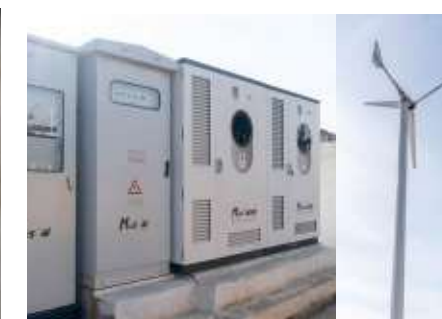
250KW/522KWH in Mespal Head quarters project
