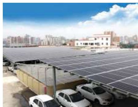
232.26KW photovoltaic carport project at Foshan Century Auto City
