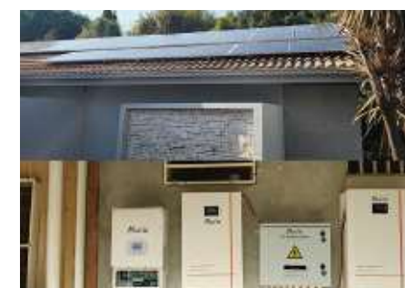
10KW solar + 20KWH lithium battery hybrid solar system in Solomon Islands
