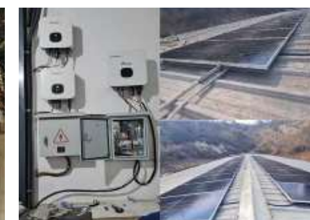
22KW on-grid solar system in Ecuador
