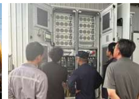
4sets 150KW/150KWH in Philippines
