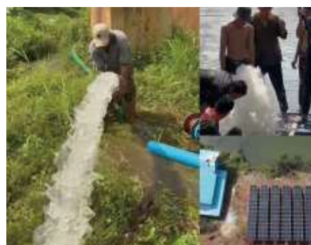
4KW solar water pump system in Philippines
